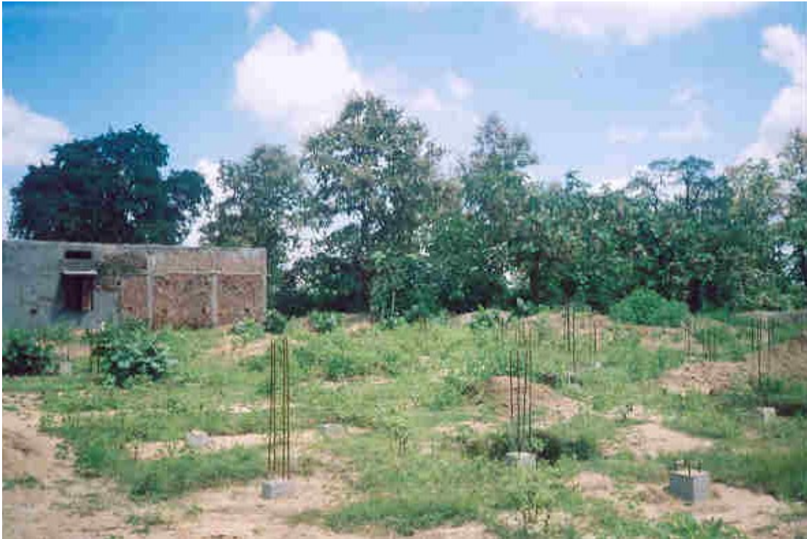
Plate 2: Delay in the construction of KGBV hostel building
